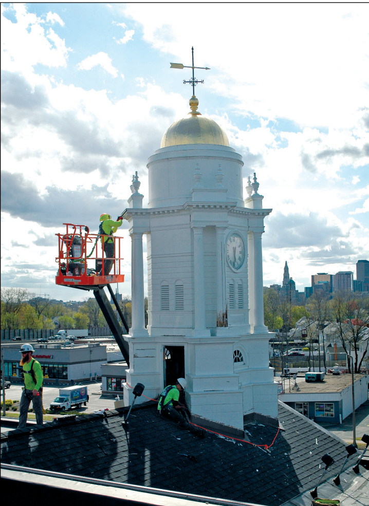
DAN, NATE AND AMERICO of P.E.S. Building Contractors of Berlin remove old caulking preparing to re-caulk the cupola atop Town Hall Wednesday.
