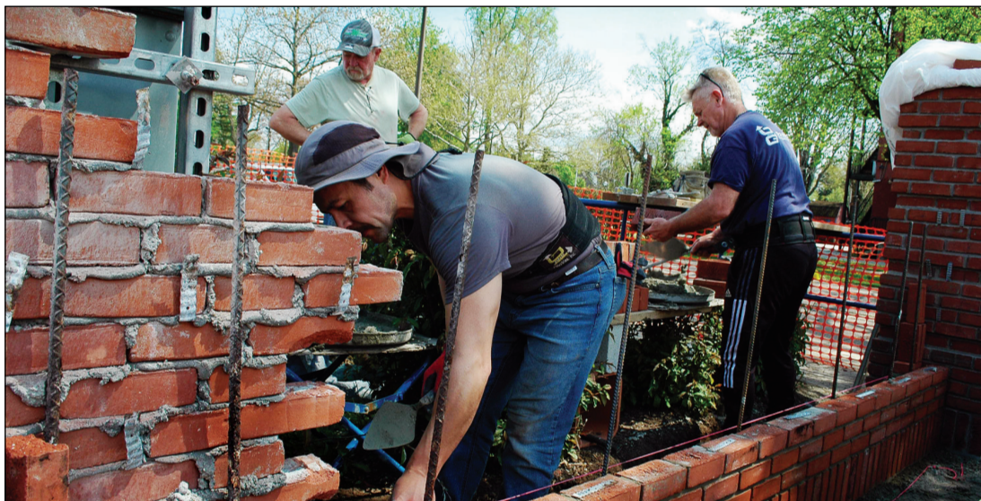
REBUILDING 'WELCOME TO EAST HARTFORD' WALL - AGAIN - Gannon Enterprises, LLC owner John Gannon, right, and masons Mick and Jose rebuild the brick wall demolished by a truck accident in February. It is the third time Gannon's company has rebuilt the wall after an accident.
