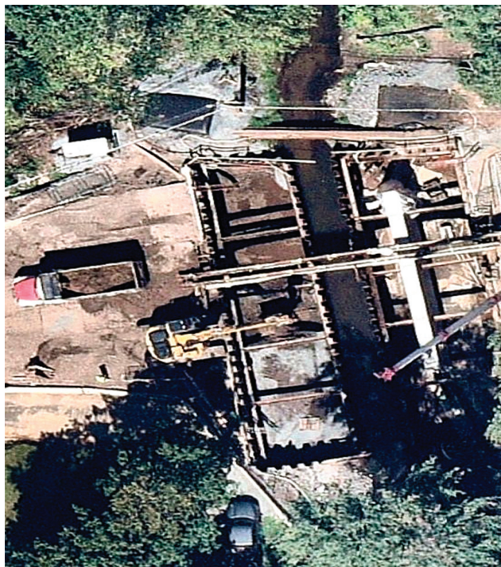
THE TOWN posted this arial photo of the work on the bridge over the Pewter Pot brook on Brewer Street. The project will not be finished until
